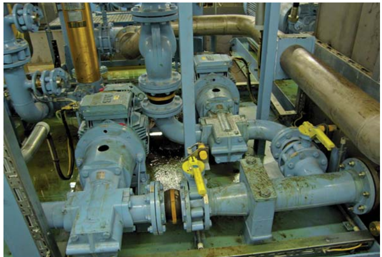
Figure 2: Hydraulic pumping unit in a steel mill
