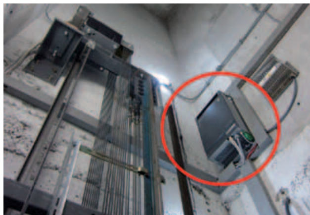
Figure 1: The inverter mounted on the top of the shaft is hard to access; the Zetadyn 3C inverter from Ziehl-Abegg is CiA 417 compliant and implements the virtual terminal interface
